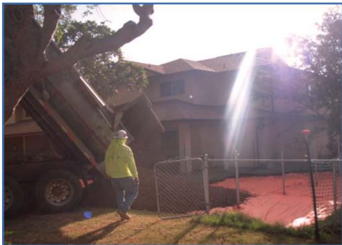
Figure 3. Backfilling clean soil on a geotextile barrier at an excavated DU at the Earhart I-2 neighborhood.
